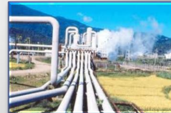
610 MW Leyte Geothermal Power Plant
