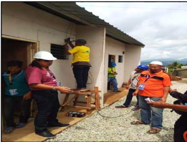
Wiring (Lighting and Convenient Outlet) for DND, DSWD and DPWH Sub offices
