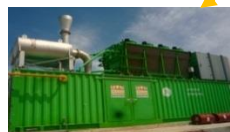
1MW DESCO (Onsite/Mine mouth Power Plant)
