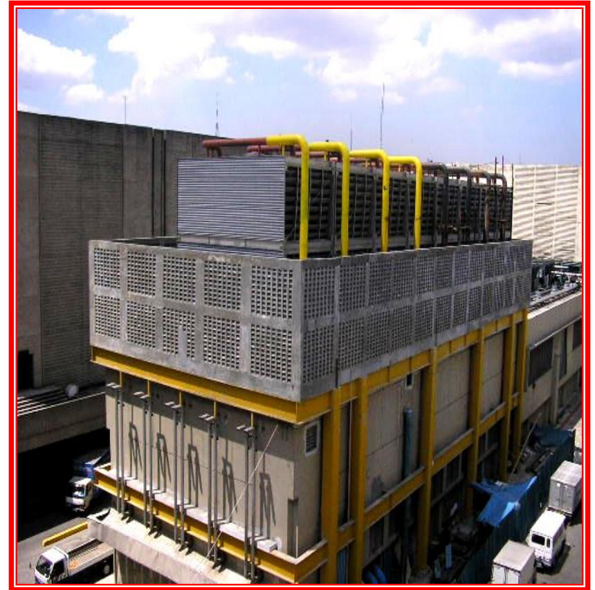
NEW COOLING TOWERS (1200 TR)
