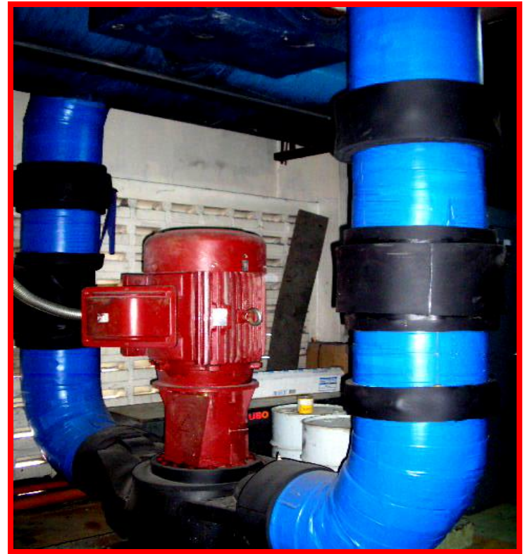
NEW PRIMARY CHILLED WATER PUMP (5 x 75kW)
