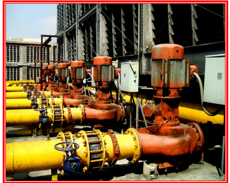
NEW CONDENSER WATER PUMPS
