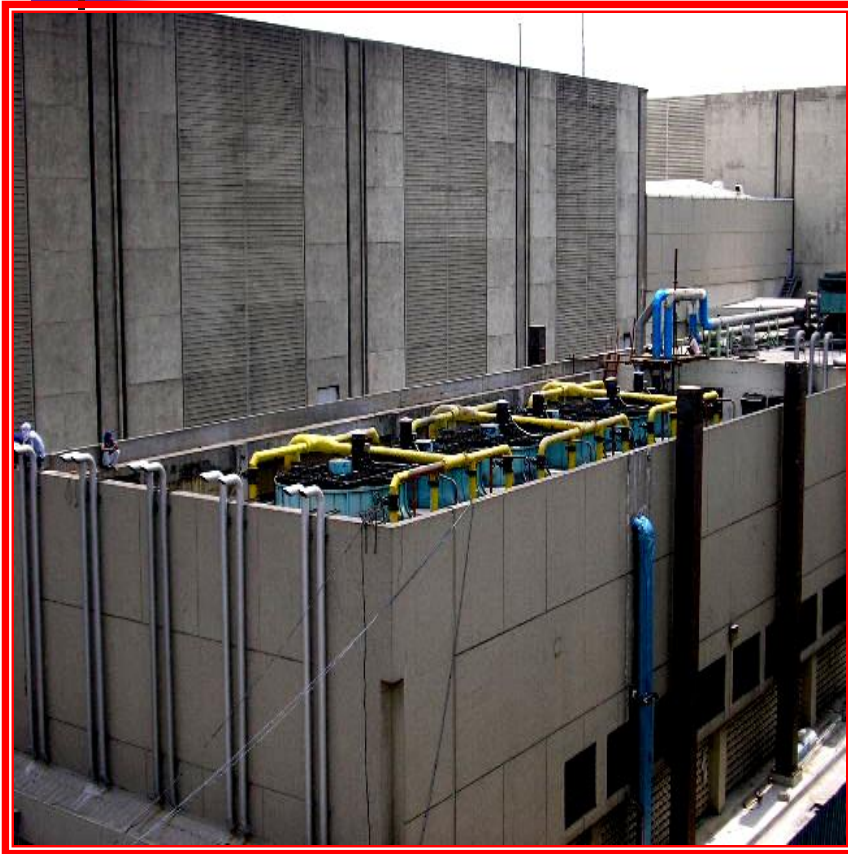
OLD COOLING TOWERS (1000 TR)
