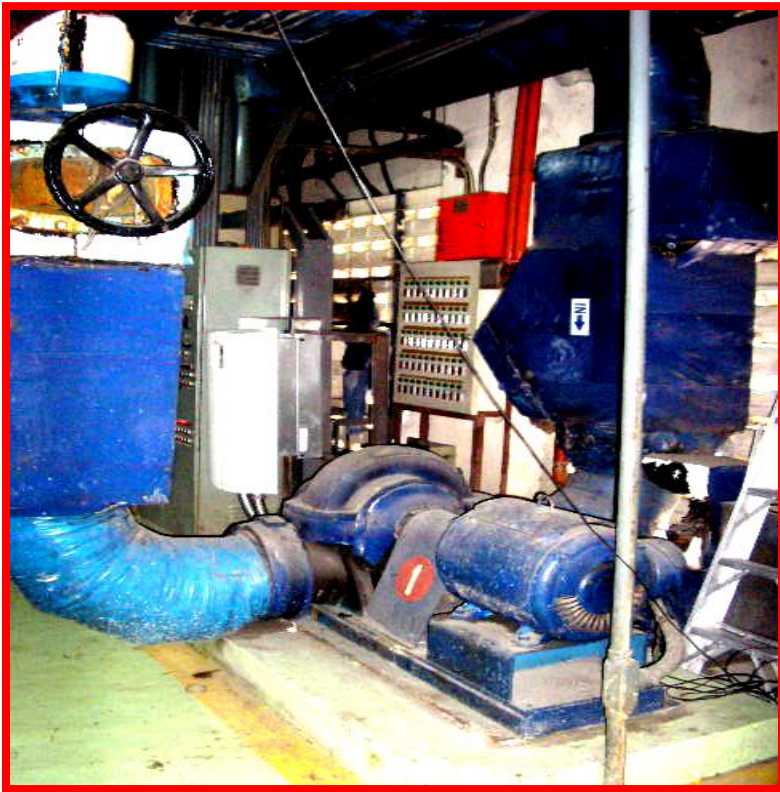
OLD PRIMARY CHILLED WATER PUMP (5 x 37.3 kW)
