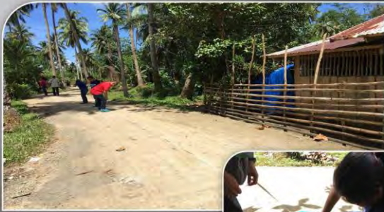
Project Title: Construction of Sta. Cruz-Badas Farm to Market Road, Municipality of Placer, Province of Surigao del Norte Project Cost: 1,899,996.20 Fund Type: DLF Power Plant: Therma Marine Mobile 2
