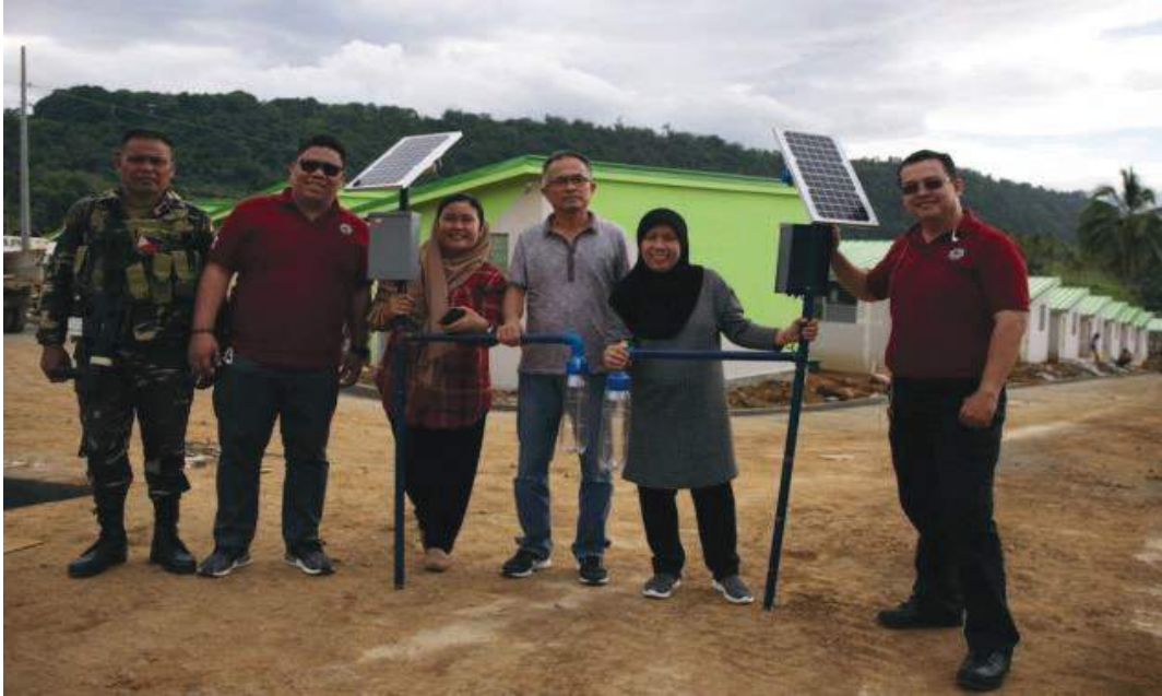
Donated solar streetlights are assembled and tested by members of the DOE, LASURECO, Task Force Bangon Marawi and the military.
